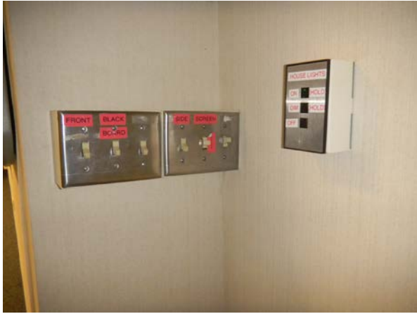
View of lighting controls
