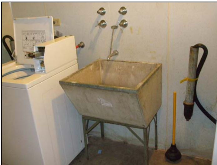
Service Sink in Basement
