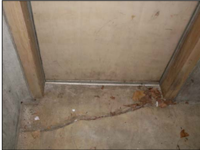
Cracks in Basement Concrete Floor Slab at Exit Door
