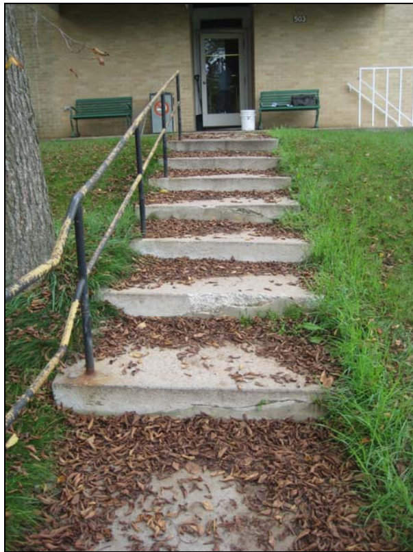
Cracks and deterioration at Concrete Stair and Paint lifting off of Steel Railing
