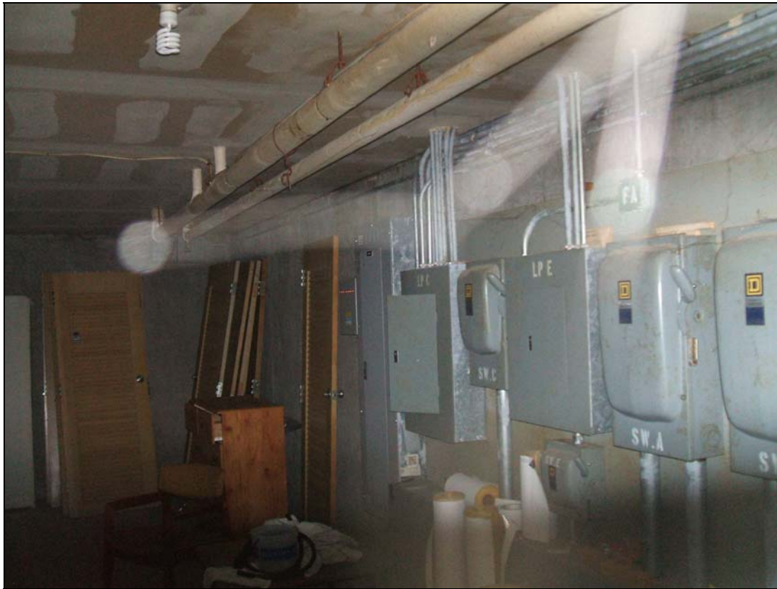
Main Electrical Room
