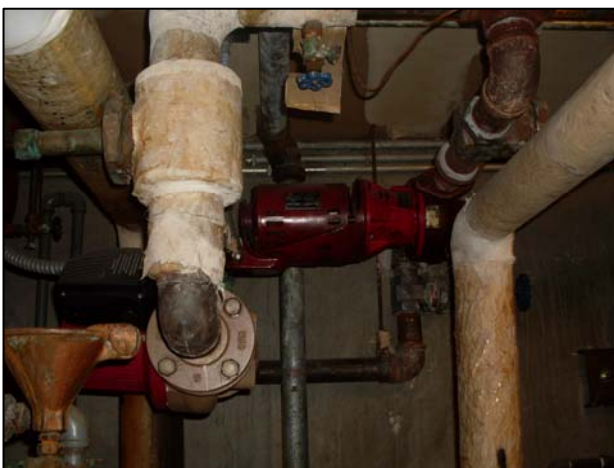
Pump and Uninsulated Steam Piping
