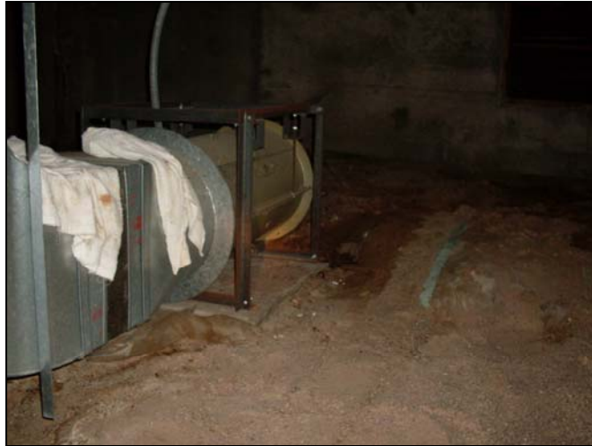
Soil Backfill at Crawl Space Appeared to be Moist during Site Visit due to Possible Pipe Leak(s)
