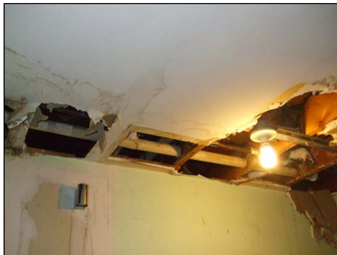
Deteriorating Drywall in Ceiling of Basement due to Possible Pipe Leak(s)
