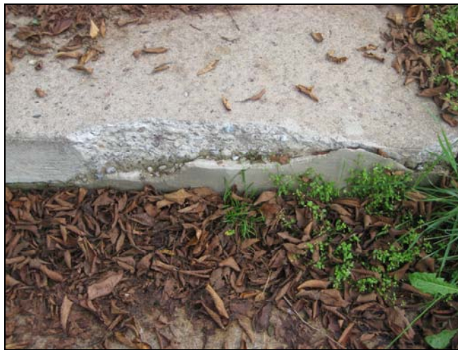
Concrete Deterioration and Cracking are occurring at this Stair Step
