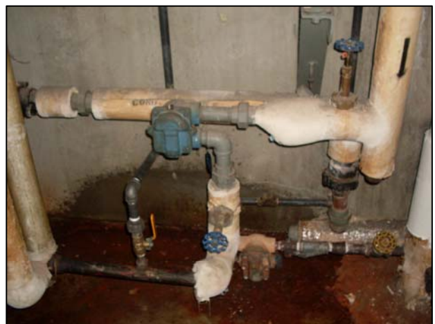
Uninsulated leaking Pipes
