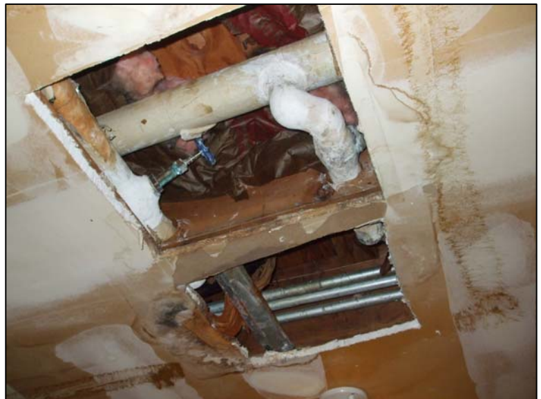
Piping in Basement Ceiling
