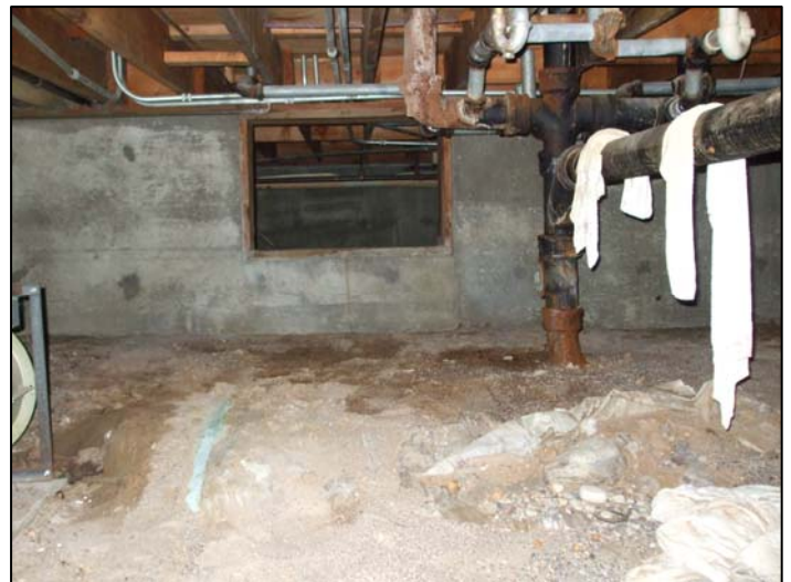
Sanitary Piping in Crawl Space below First Floor
