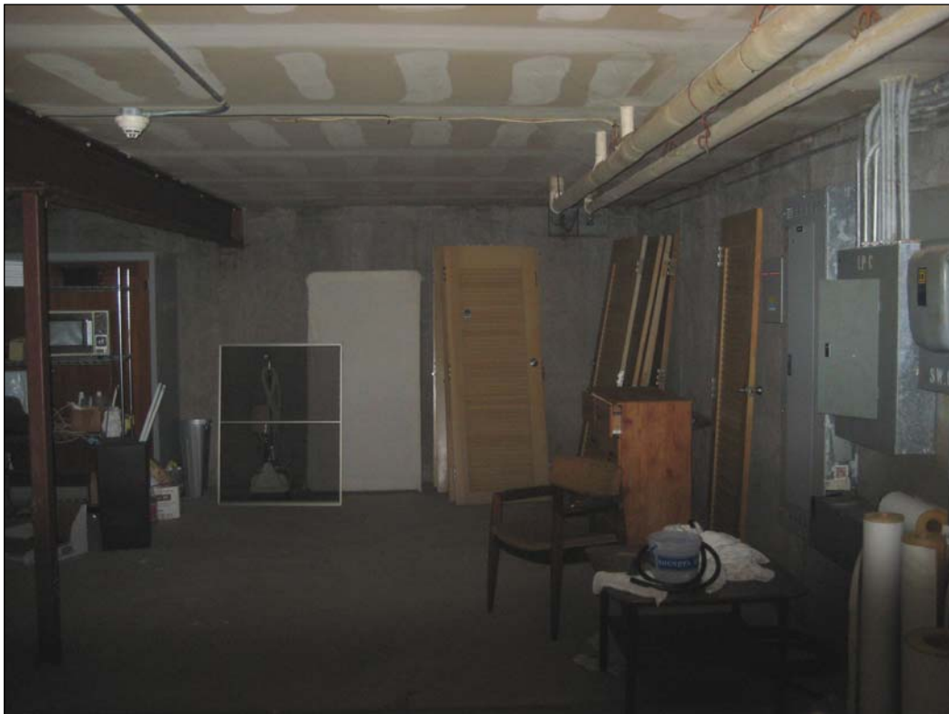
Storage/Electrical Room in Basement Level
