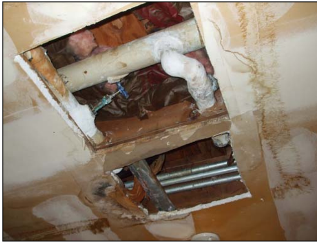
Holes in Floor Joists are not in a suitable Location from Bottom Edge of Members and are close Together
