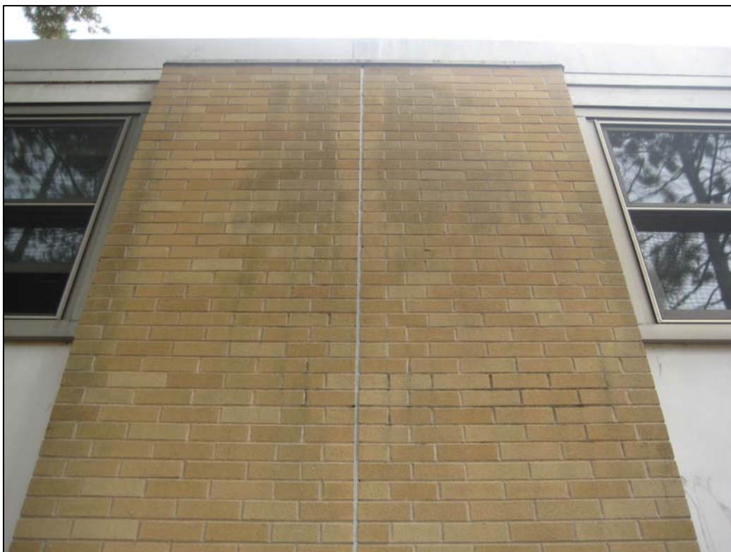
Typical Staining of Brick found around the Building's Exterior
