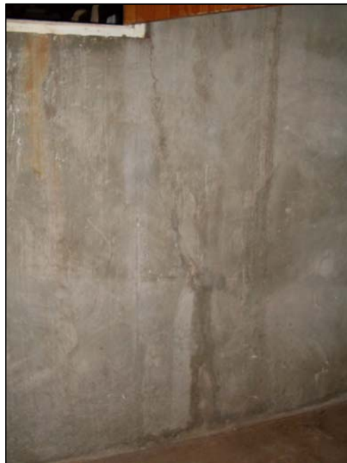
Cracks in Crawl Space Concrete Foundation Wall
