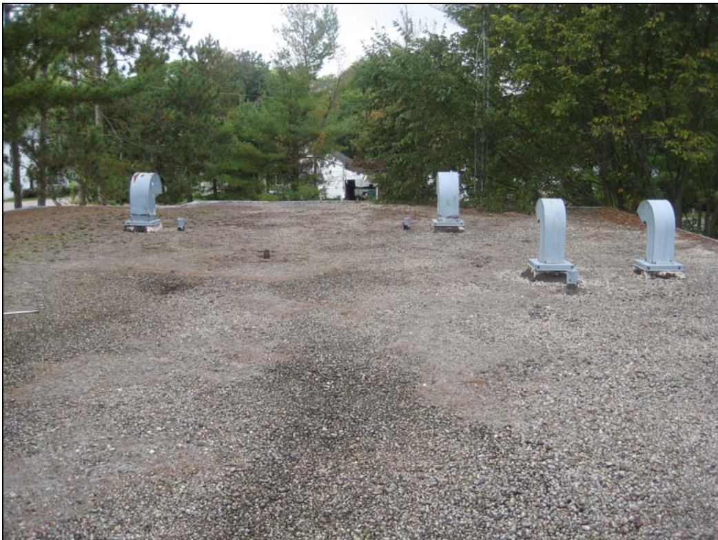
View of Roof and Vegetation Growth
