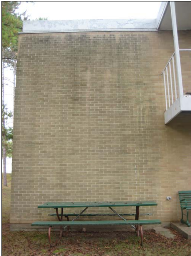
Roof Drainage Problem causing Staining on Brick Veneer
