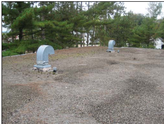
Plant Growth and Standing Water on Roof
