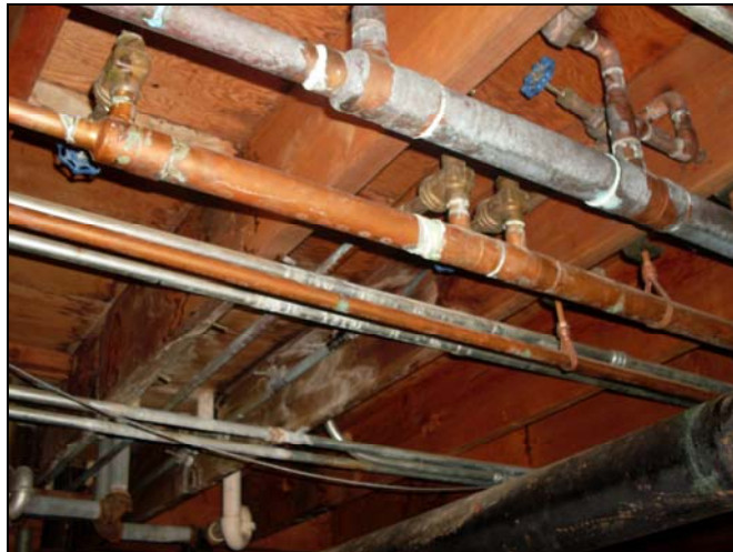
Severe Water Stains and Possible Rotting of Floor Joists above Crawl Space due to Possible Pipe Leak(s)
