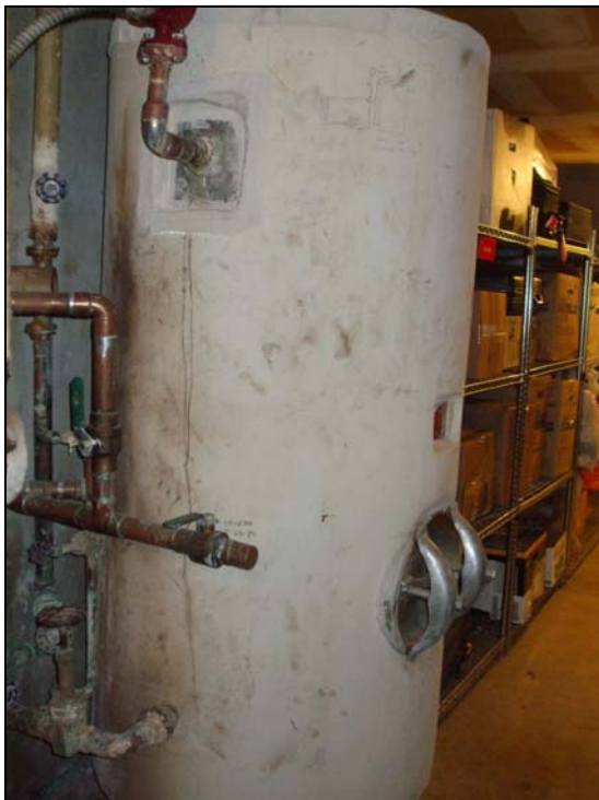
Hot Water Storage Tank in Basement
