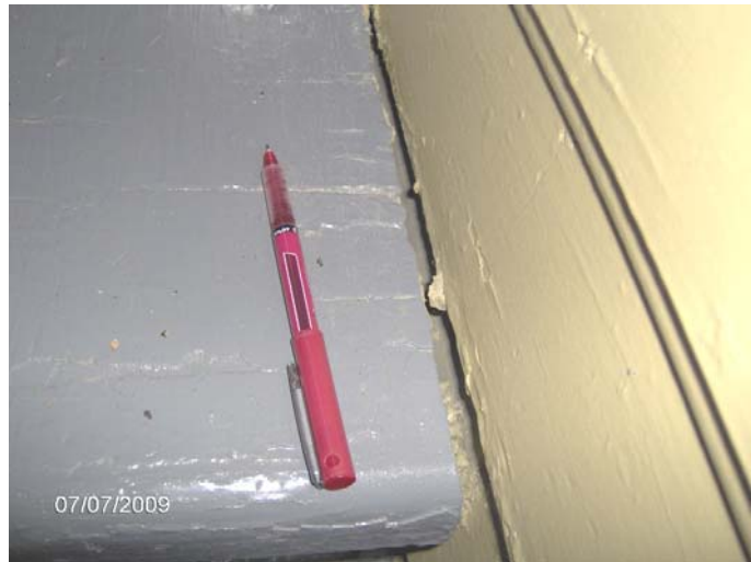
Image 15: Gap created between stair and building wall due to stair rotation.
