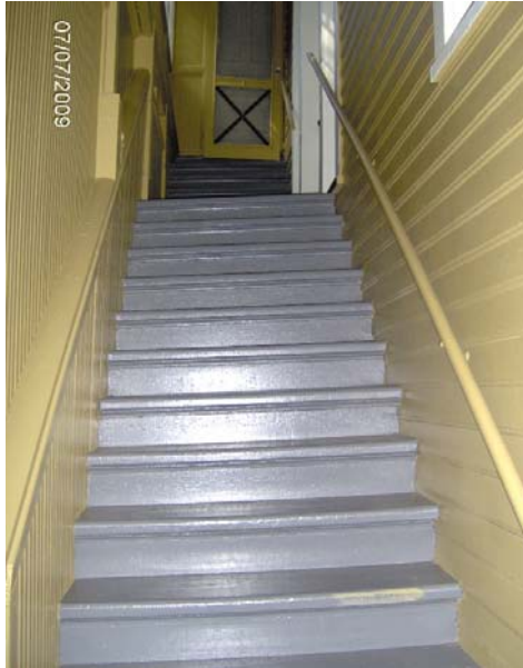
Image 14: South stair has rotated away from the building.
