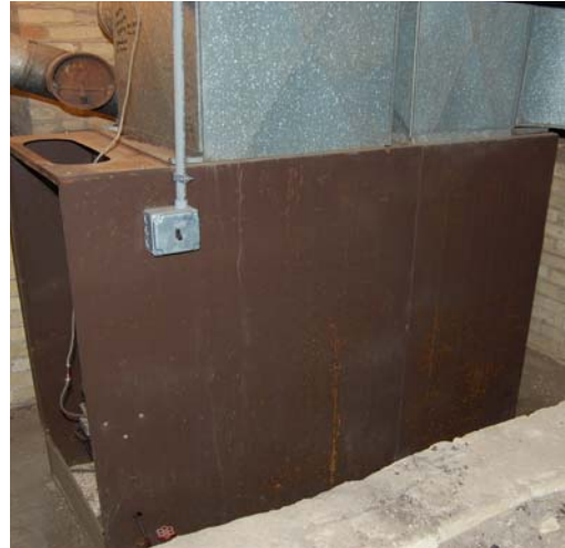
Existing oil fired furnace installed in 1986-87
