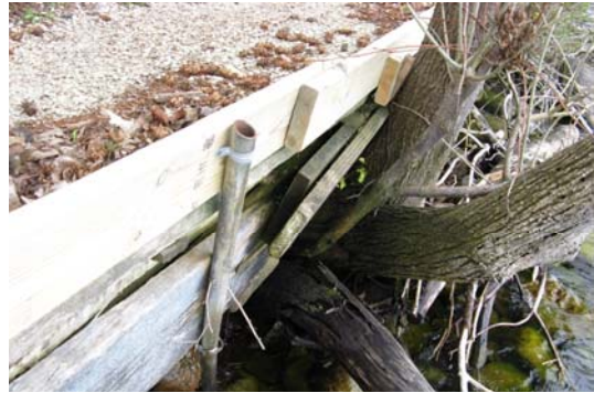
Temporary repairs installed are not adequate to stop the lakeshore erosion that is damaging the path in some locations.
