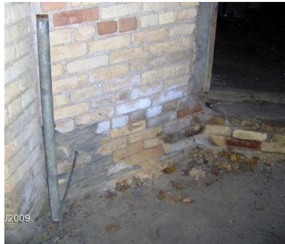
Image 2: Basement wall patched with cementitious material.
