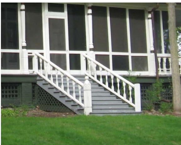
Image 5: Original handrail baluster is missing and replaced by simple 6x6
