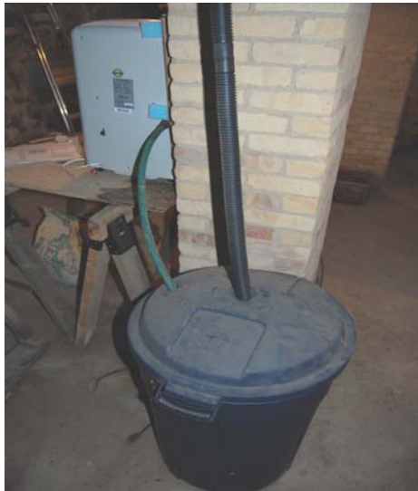
Sump pump located on floor in basement
