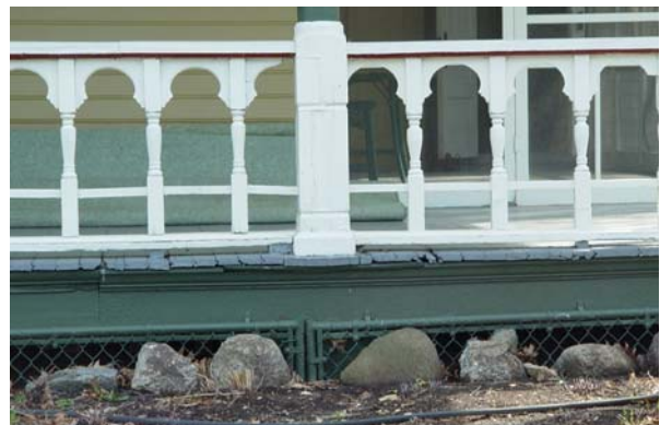
Image 2: Porch decking shows signs of decay on the ends in several places
