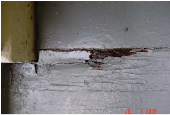
Image 3: In some areas decay in the porch deck has resulted in soft spots (see diagram on p. 51 for locations)
