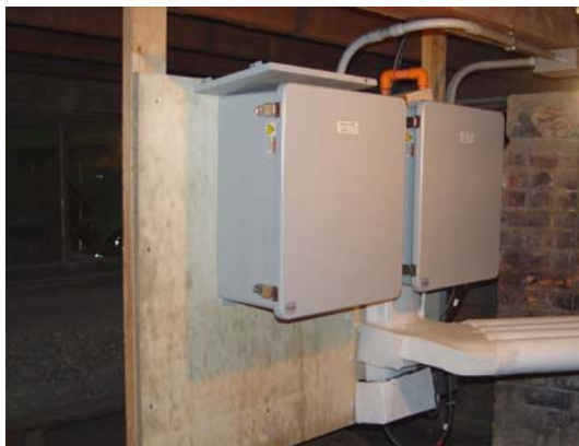
VESDA air sampling fire detection system installed in 2006 in the crawl space.
