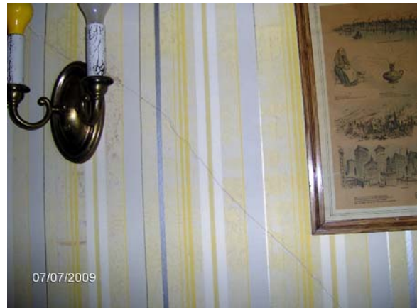
Image 7: Diagonal cracks in third story walls
