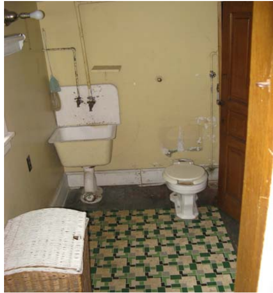
Image 14: Example of fixtures in disrepair, as seen in the bathroom off of stair landing between the 2 nd & 3 rd floors.
