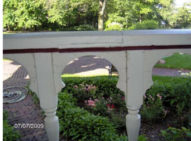
Image 13: Splice in porch railing
