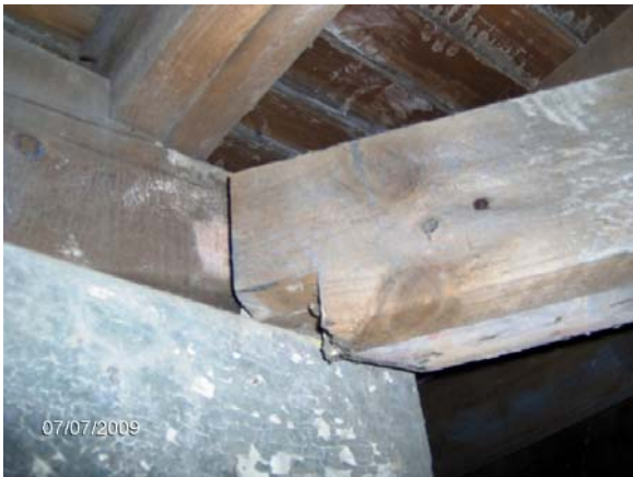
Image 9: Insufficient porch beam bearing
