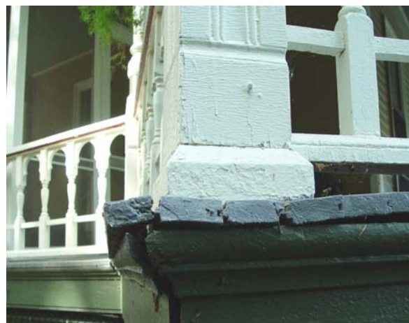
Image 6: This area on the northeast corner of the porch shows deck boards and trim detaching from the structure
