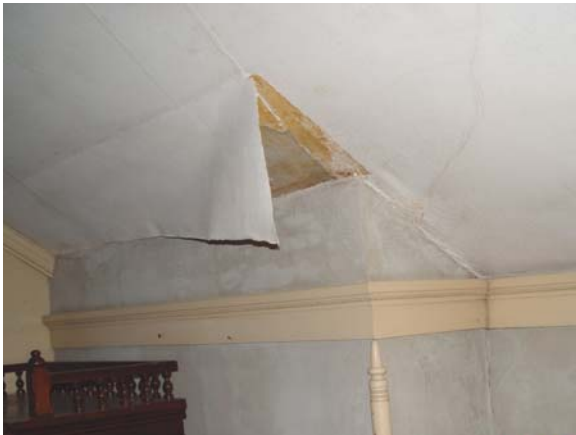
Image 11: The original burlap wall covering is peeling in several areas, although typically not as severely as this example in the third floor Gray Room.
