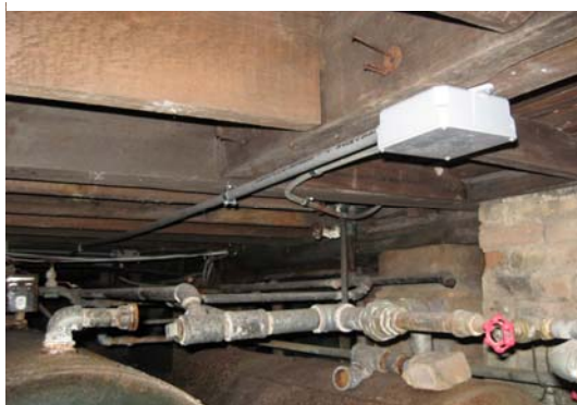
The connection between new crawl space wiring and original wiring. All crawl space wiring was replaced in 2006.
