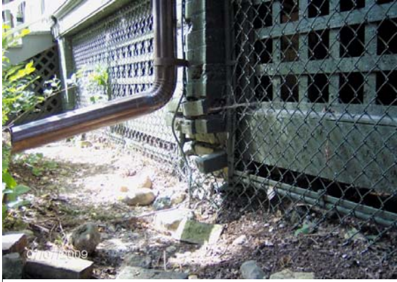
Image 8: Damaged porch pier (see noted plan diagram p. 50)
