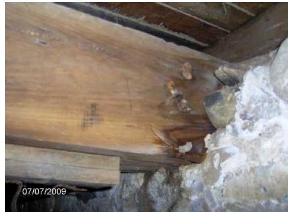
Image 5: Deterioration at the end of floor beam where it is bearing into the masonry wall.
