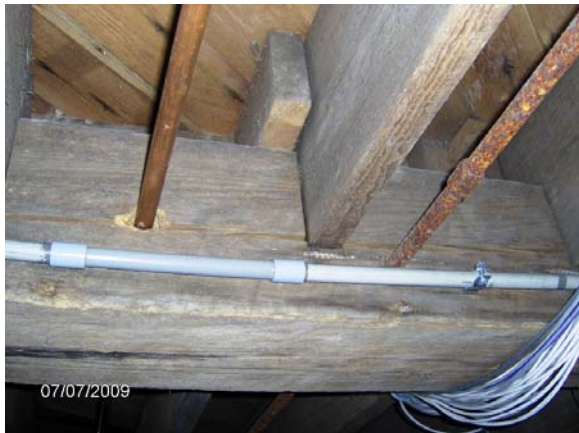
Image 4: Notches, checks and holes are located at the same depth in the floor beams.
