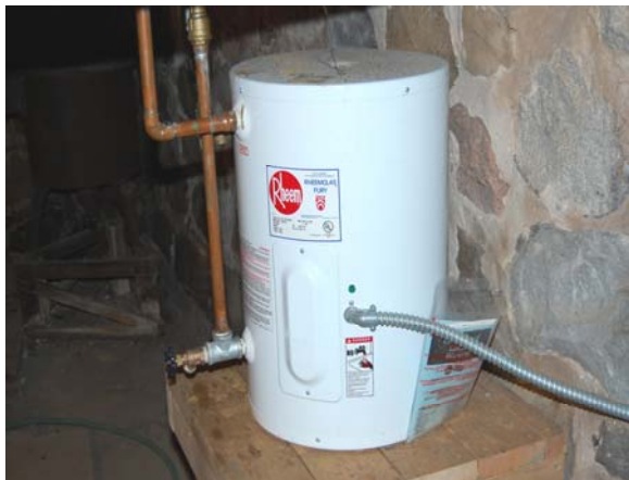
Water heater serving kitchen sink
