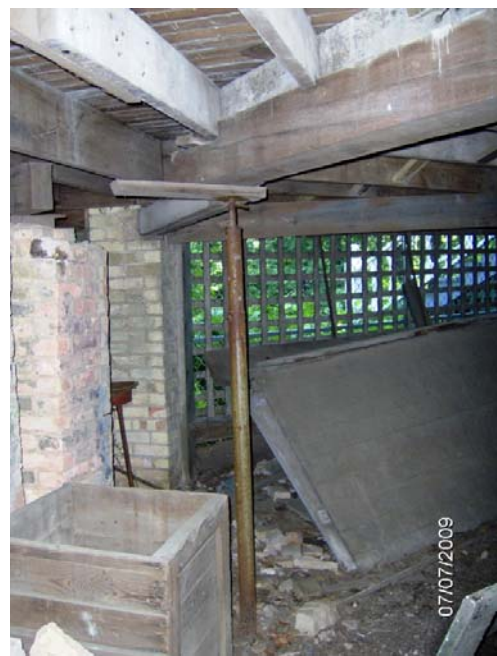
Image 10: Adjustable pipe column supporting porch framing
