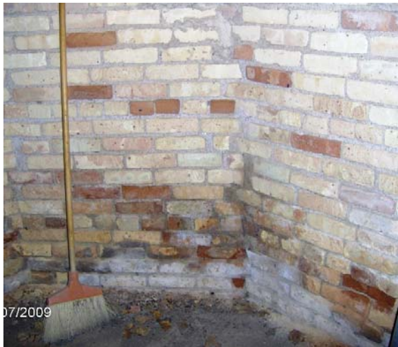
Image 1: Deteriorated basement wall (see noted plan diagram pg. 50)
