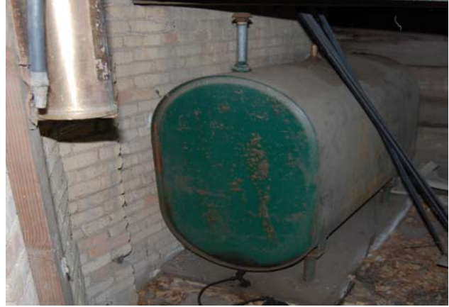
Existing oil storage tank
