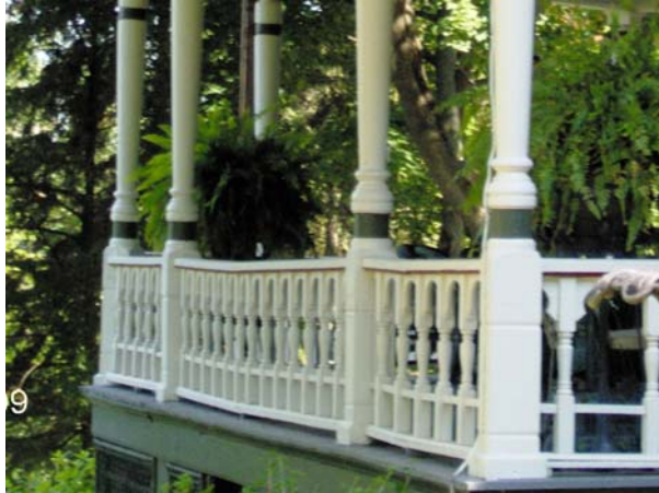
Image 12: Sagging porch railing
