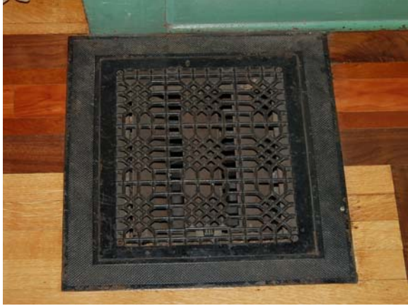
Floor grate for central heating system
