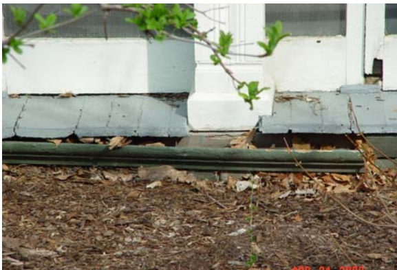
Image 1: Example of trim piece that has detached from the porch
