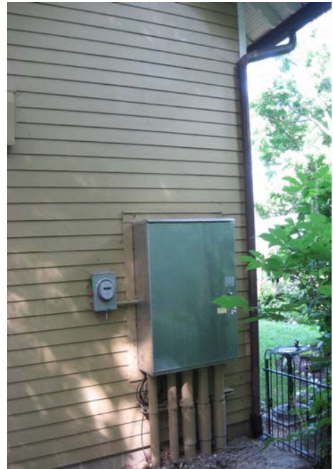
New underground service at Visitors Center outbuilding installed in 2006
