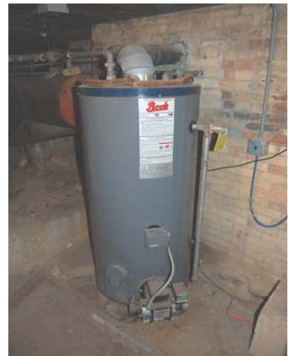
Fuel oil fired water heater
