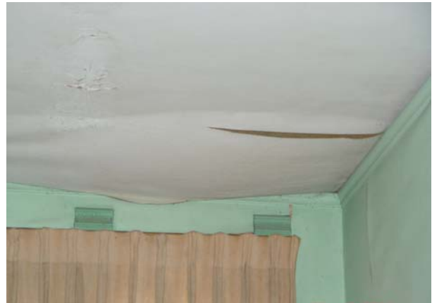
Image 12: This spot on the ceiling above the main staircase also shows damage to the covering.
