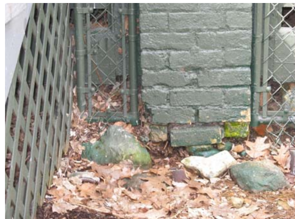
Image 10: Eroded mortar joints and dislocated bricks are a fairly typical condition found on the base of the exterior piers.
