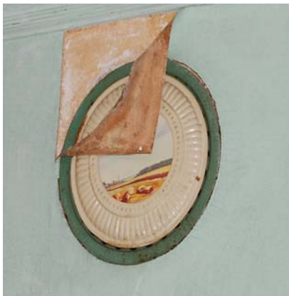
Capped flue pipe of removed wood burning pot belly stove
