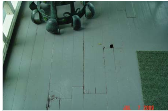
Image 4: Another example of porch floor boards that show signs of decay
