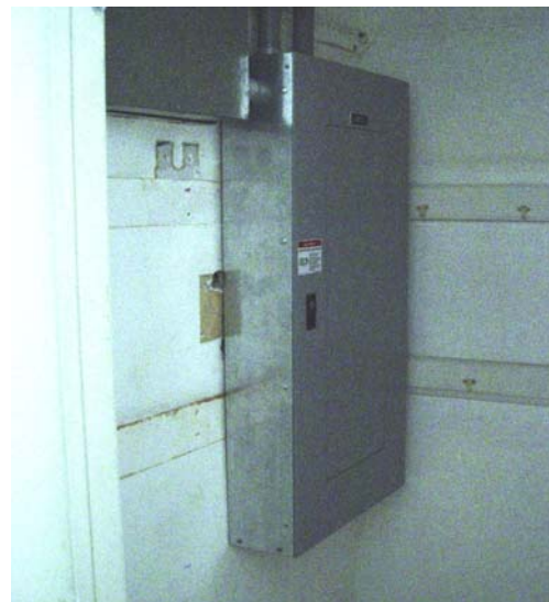
On the second floor a new circuit panel replaced an early plug-fuse panel in 2006.
