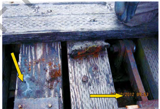
Asbestos Sample 02, coating on south tie PCB Sample 002, grease south end
