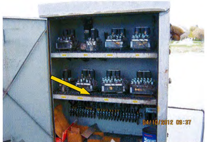
Inside electrical box, assumed ACM electric component Inside electrical box, PCB Sample 001 of shelf residue
