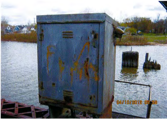
Electrical box on east side, north of east shed
