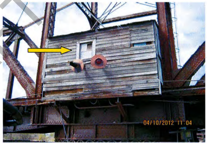
Assumed ACM window glaze on east shed
